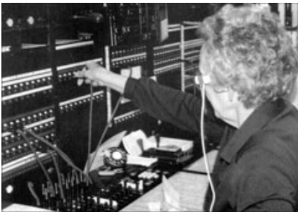
Operator Erma Campell was photographed as she worked the switchboard.
